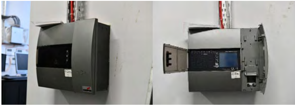
Fire Alarm Control Center
