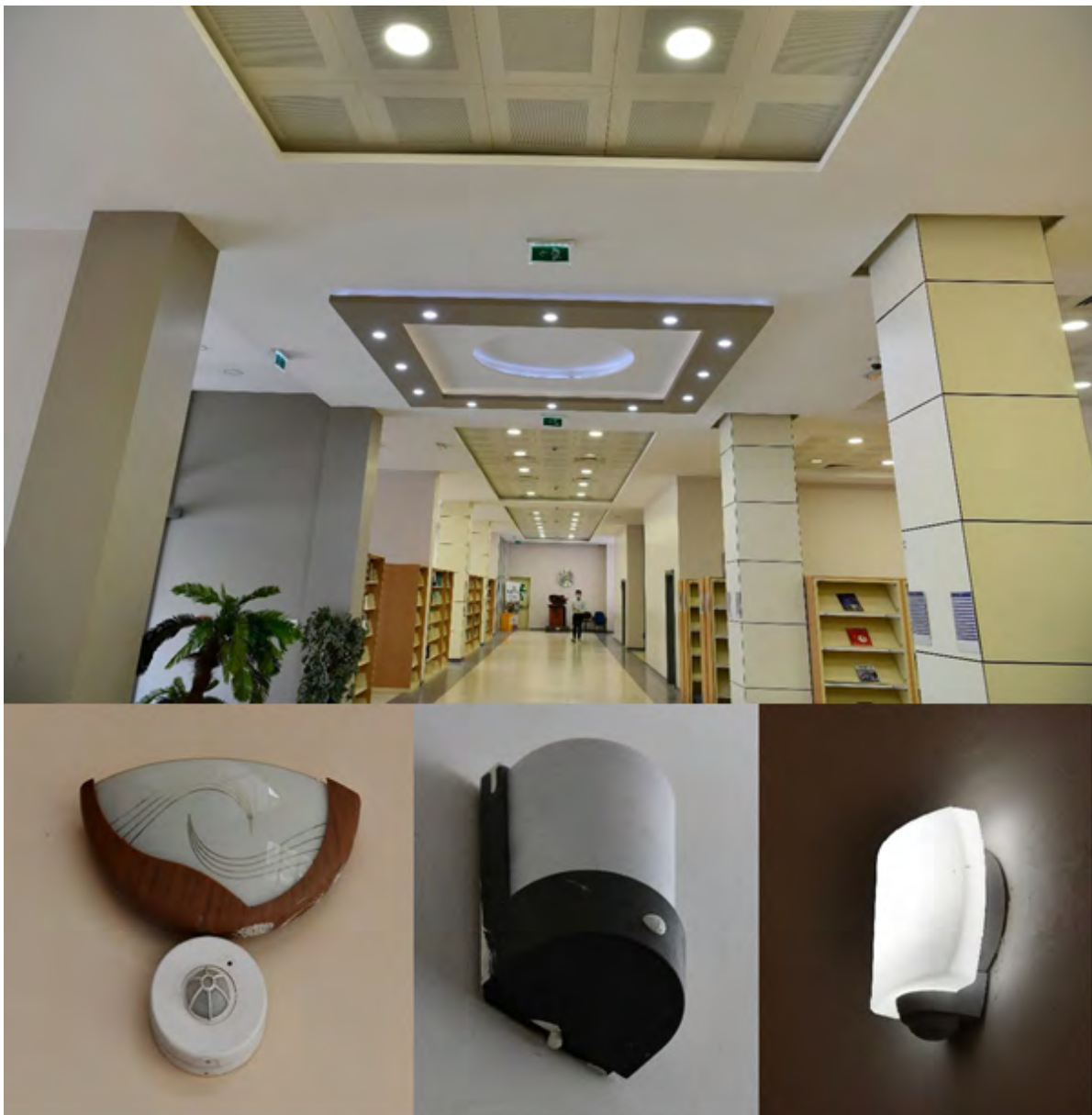
Figure 25: Use of LED lighting and lamps with light detection
