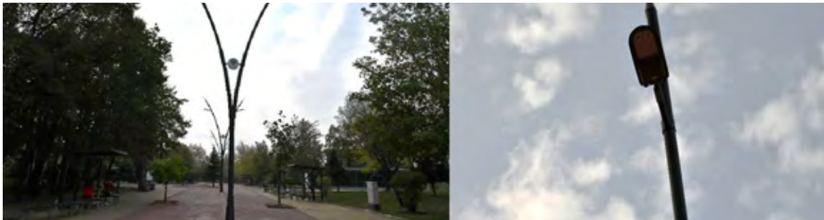
Figure 81: Solar Street Lamps
