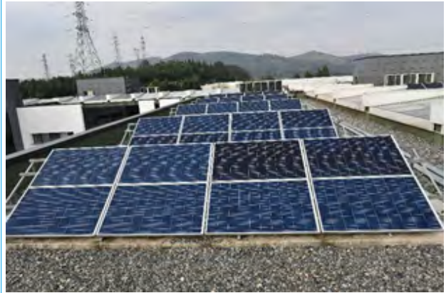
Solar Energy Panels
