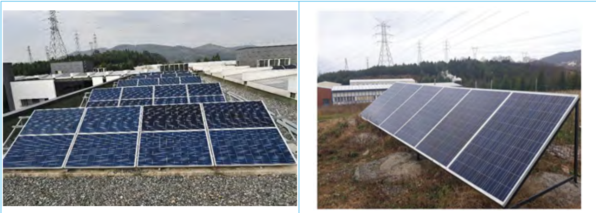
Figure 29: Roof Solar Panels
