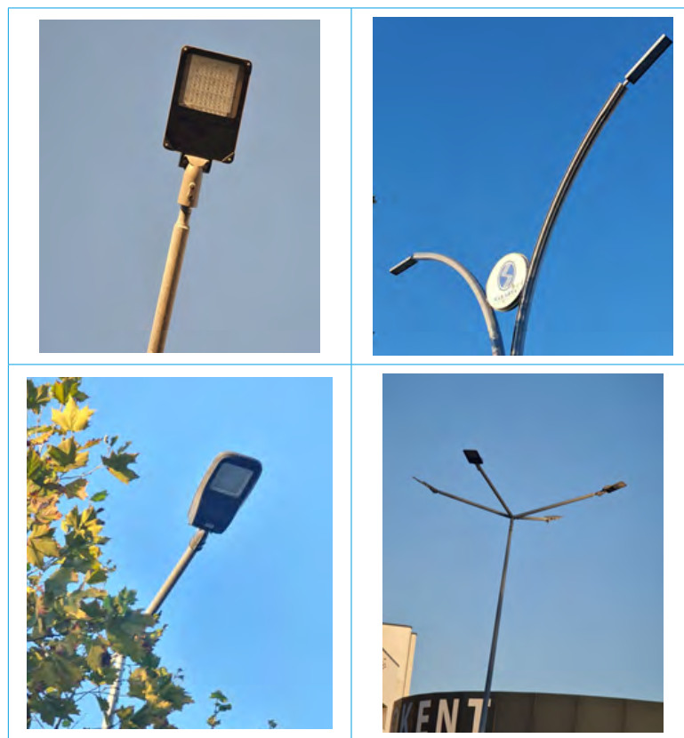
Figure 31: Solar street lamps
