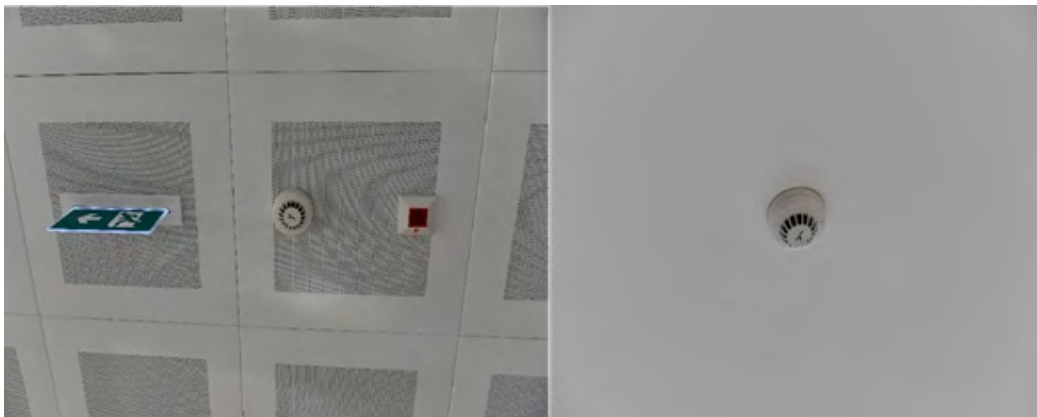
Automatic Fire Alarm Sensor
