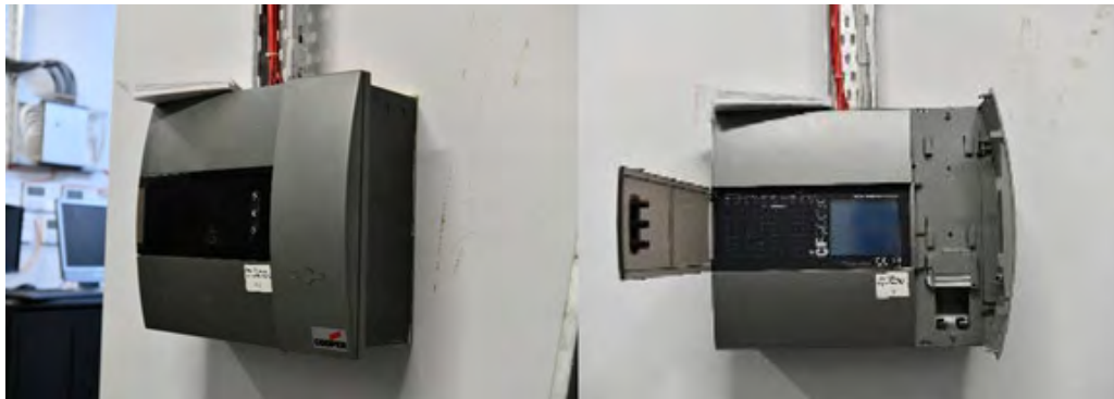
Fire Alarm Control Center
