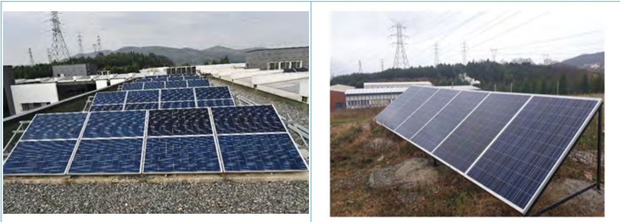
Figure 27: Roof Solar Panels
