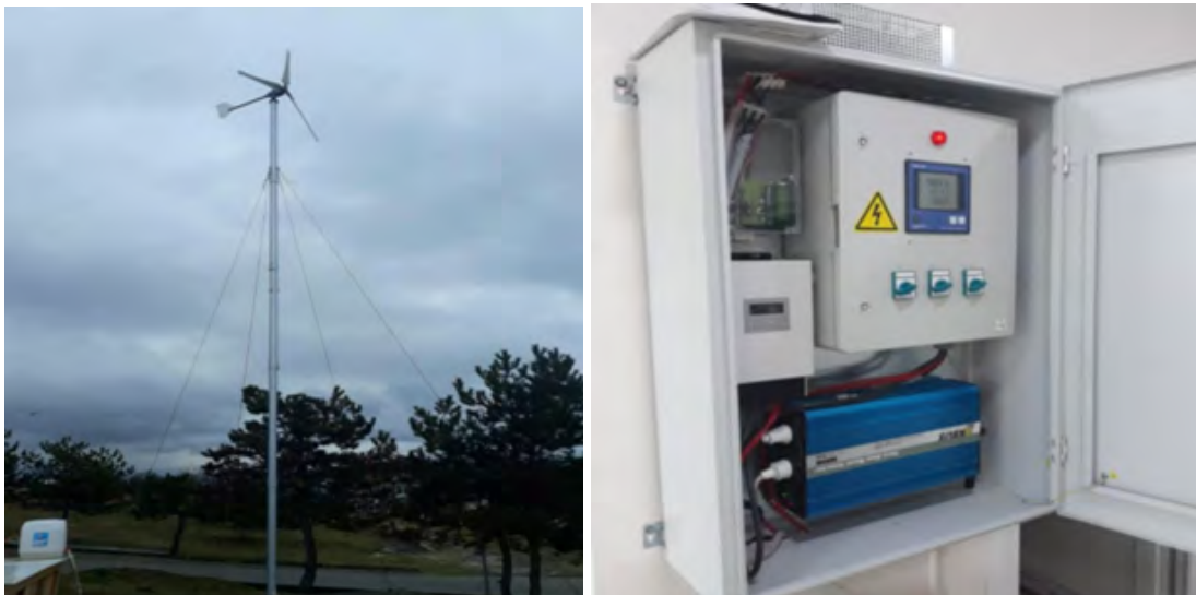
Figure 28: Wind Turbine and Control Panel of Wind Turbine
