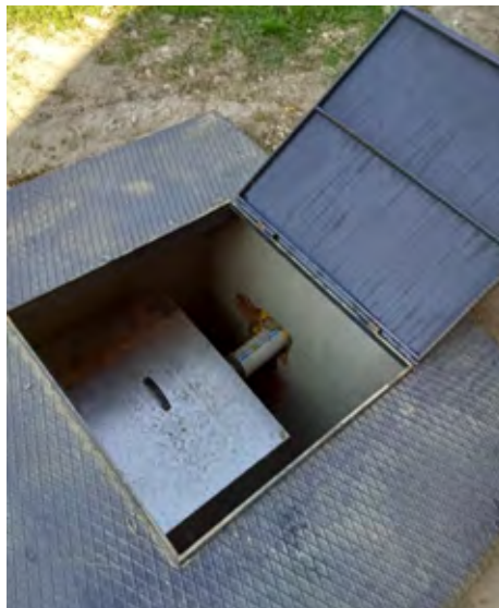
Figure 50: Oil filter for organic waste
