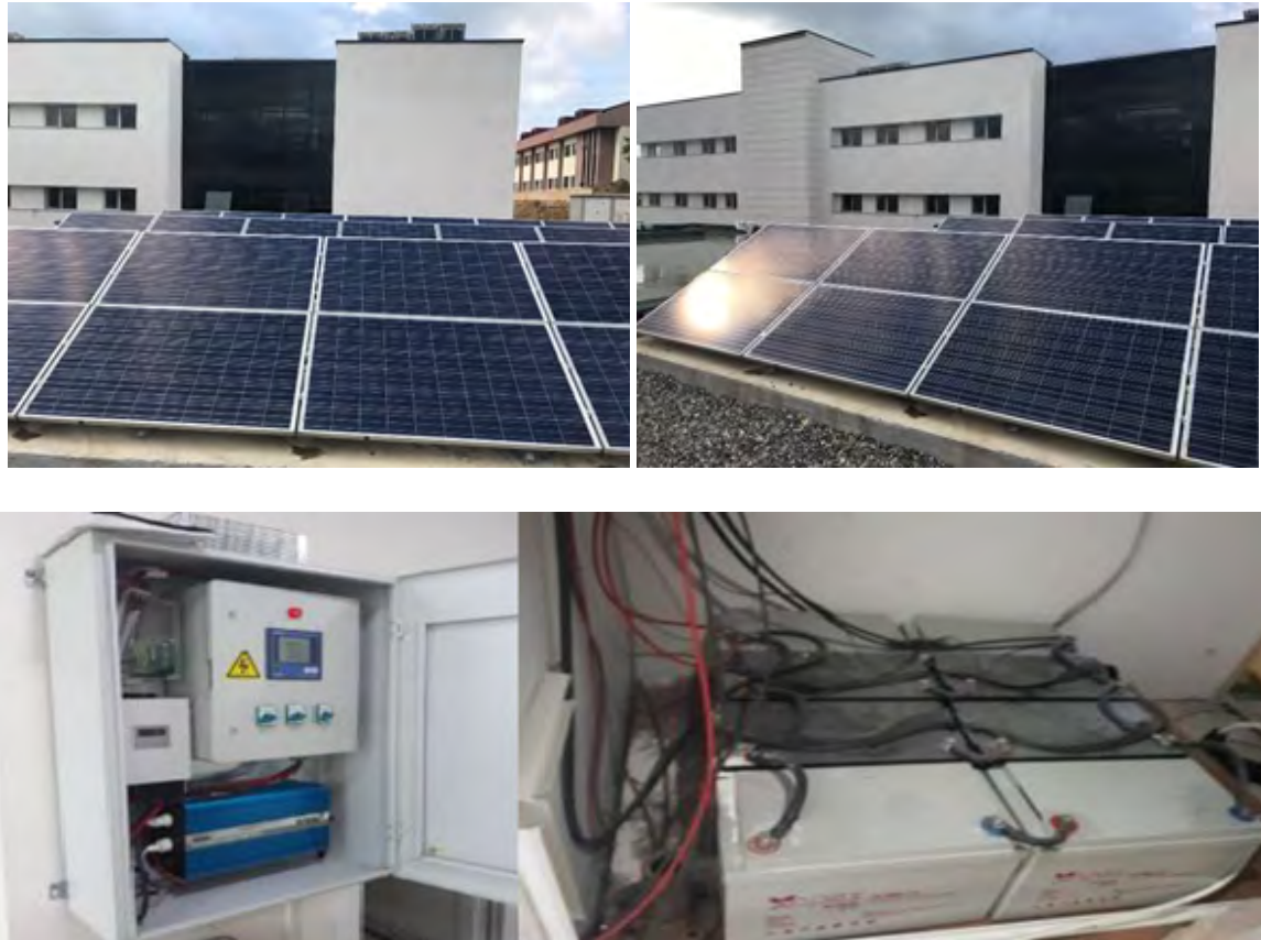
Figure 32: Energy Management Tools
