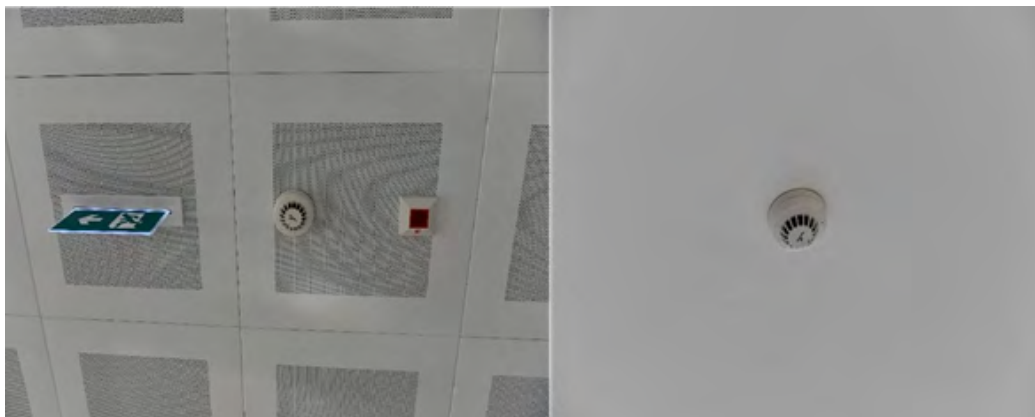
Automatic Fire Alarm Sensor
