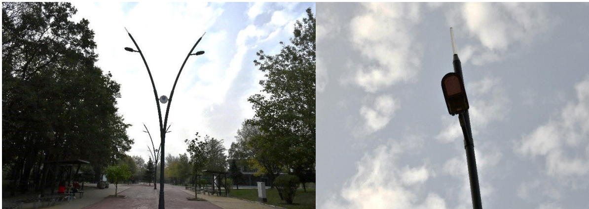
Figure 59: Solar Street Lamps
