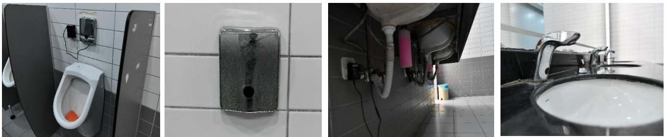
Figure 42: Water Efficient Appliances Usage
